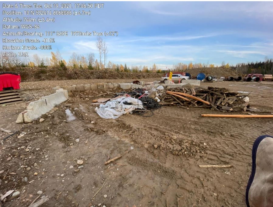
Photo 19. Mixed waste, including food waste, stored on the ground within Parsnip MUS. Signs that birds accessing this waste were observed while EAO C&E was on site.
