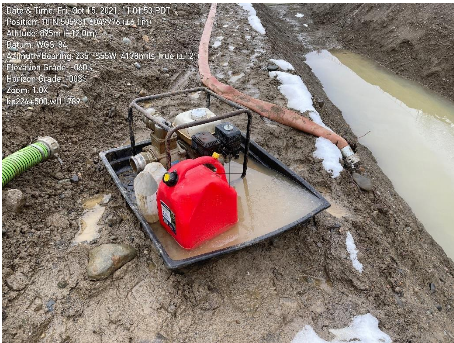
Photo 33. KP224+500. Secondary containment beneath pump at capacity with water.
