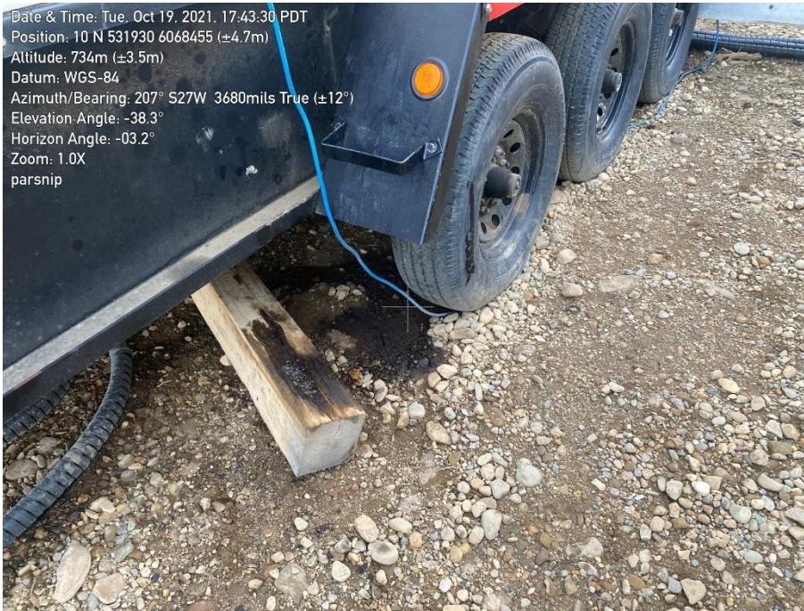
Photo 45. Leak to ground beneath active generator at Parsnip MUS.
