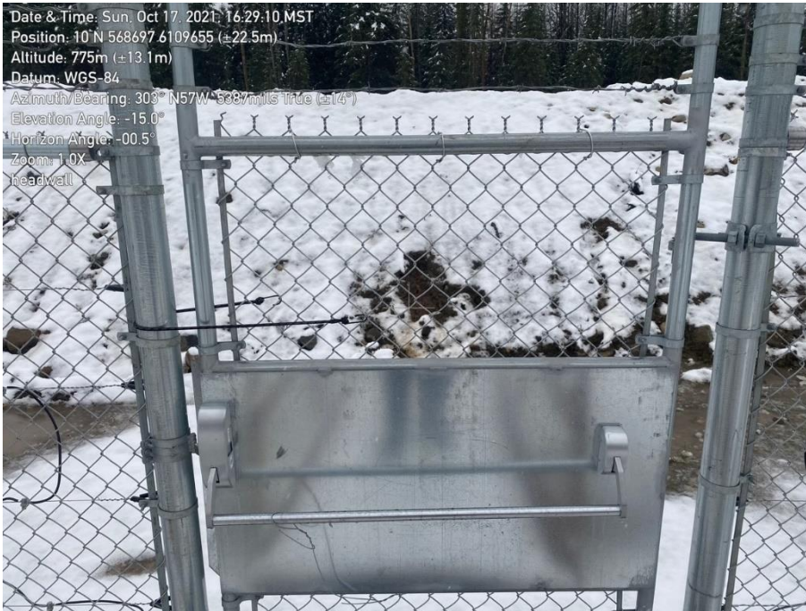
Photo 44. Example of man-gate secured closed using bungy cord – Headwall MUS.
