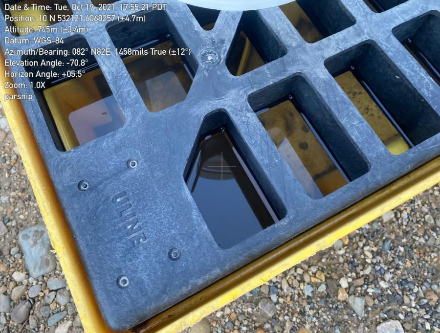
Photo 36. Close up of spill tray seen in photo above. Spill tray near capacity with rainwater.
