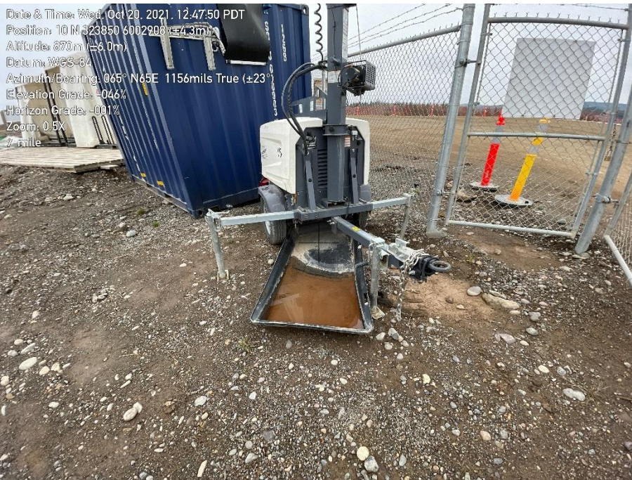
Photo 37. Secondary containment on angle and at capacity with water.
