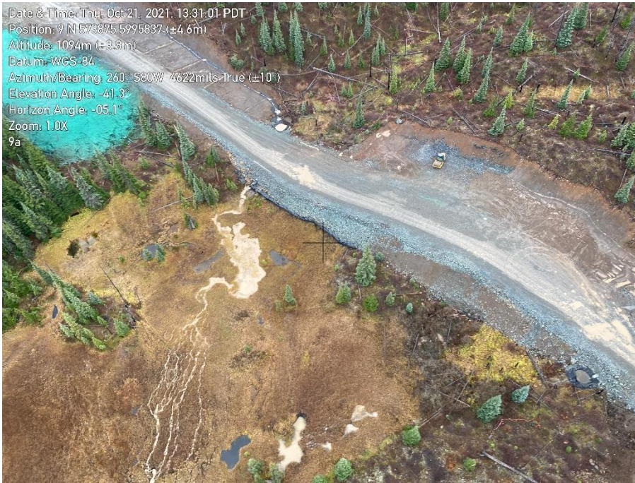
Photo 11. Near KP 600+500. Sediment laden water leaving ROW and discharging to wetlands downslope.
