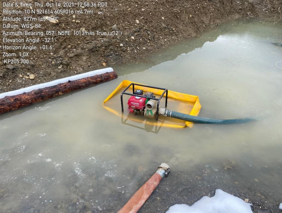
Photo 32. KP205+700. Pump and containment submerged in water.
