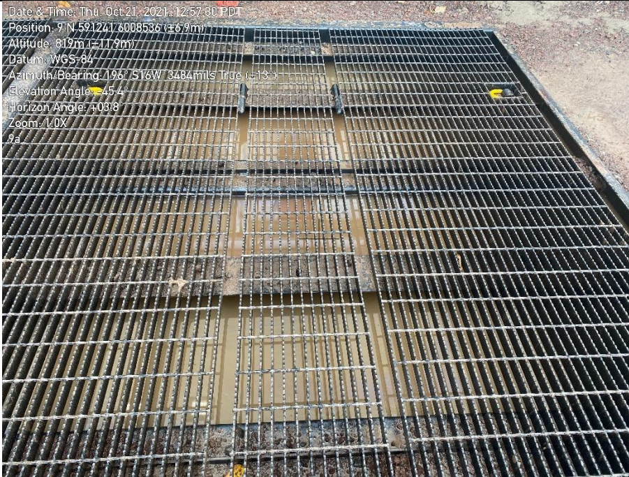
Photo 40. Containment beneath vehicle parking area at fuel island near capacity – MUS 9A.
