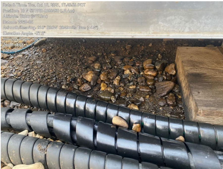
Photo 46. Close-up of an active leak to ground beneath an active generator at the Parsnip MUS.
