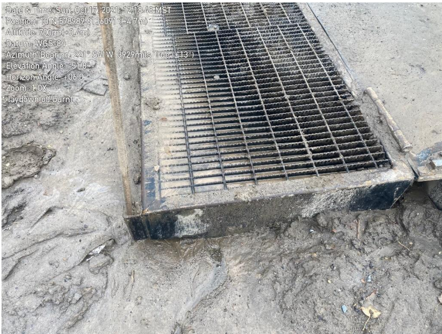
Photo 42. Close up of location in red circle in above photo where containment overtops.
